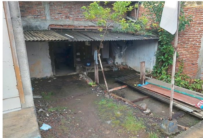
Figure 2. Condition of Houses Affected by Rob Floods in the Kaligawe Region, Semarang
