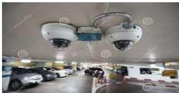
Fig.6 CCTV in Parking Zone
